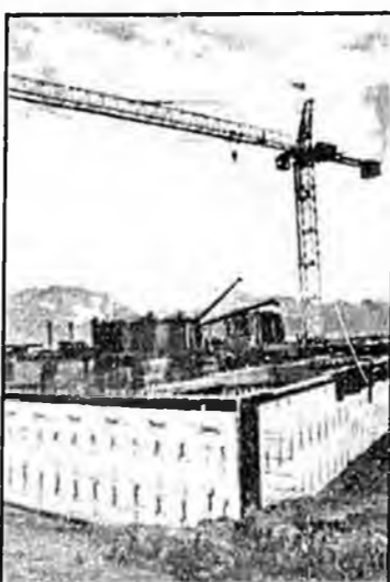
Construction of the Alaska SeaLife Center in Seward got underway this summer with opening scheduled for May 1998.
