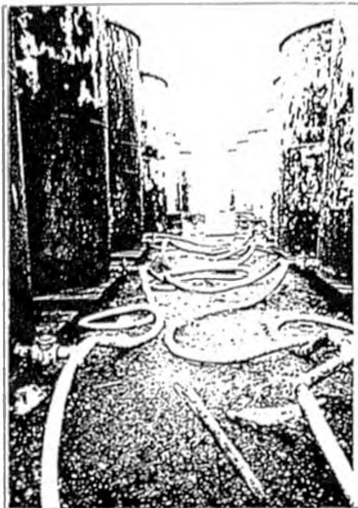
Photograph A.1 Severely corroded tanks connected by rubber hose. Evidence of fuel spillage throughout area.
