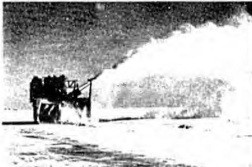
PEAK UTILIZES SNOW BLOWERS TO MAINTAIN ICE ROADS, AIRPORT RUNWAYS, AND GRAVEL ROADS AND PADS FOR SEVERAL CLIENTS ON THE NORTH SLOPE.
