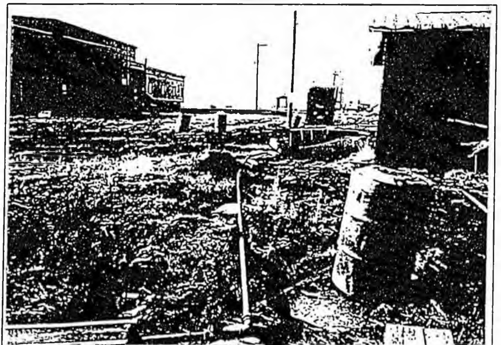
Photograph A.10 Faulty piping system reportedly broke during winter, spilling an estimated 50 gallons of fuel.
