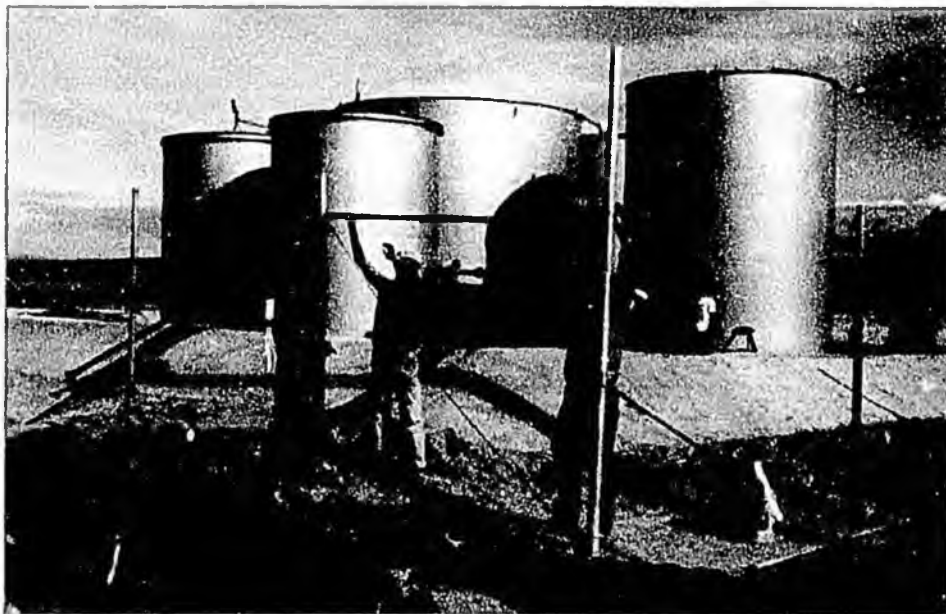
CONSTRUCTION TOOK PLACE LAST SUMMER ON NEW, ENVIRONMENTALLY SOUND FUEL STORAGE FACILITY FOR GOLDMIN.
