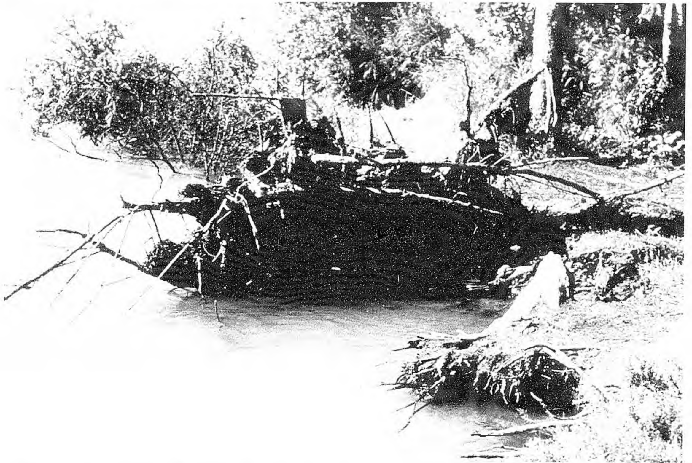
Photo # 8 Erosion of undercut banks -- Kenai River
