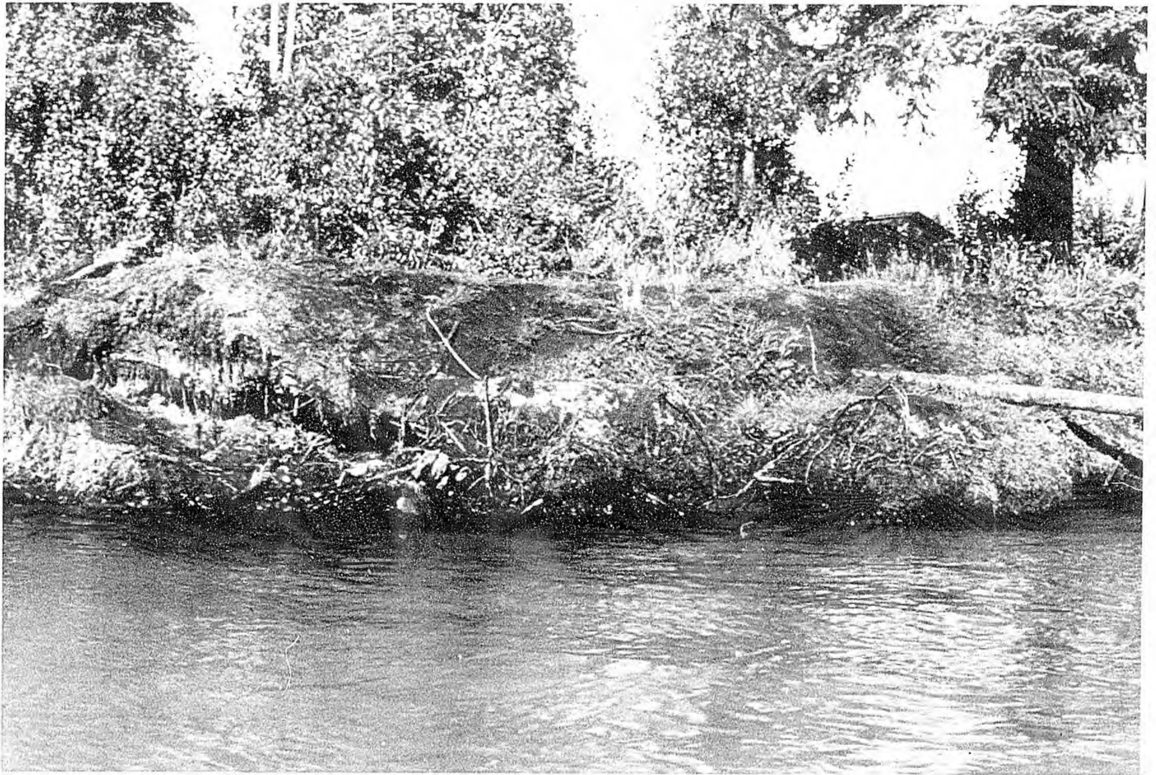
Photo # 7 Sport fishing access and erosion of undercut banks -- Kenai River
