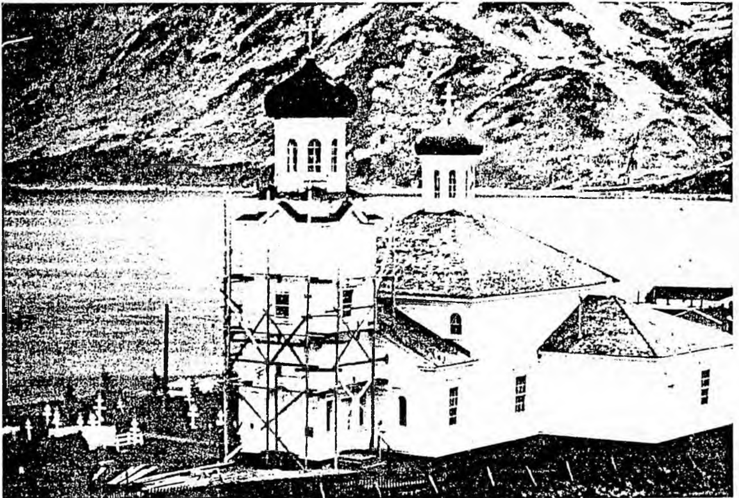
Although maintenance work is done on a continuing basis, severe weathering conditions and structural problems threaten the long-term preservation of this magnificent church. Photo: CCC Architects
