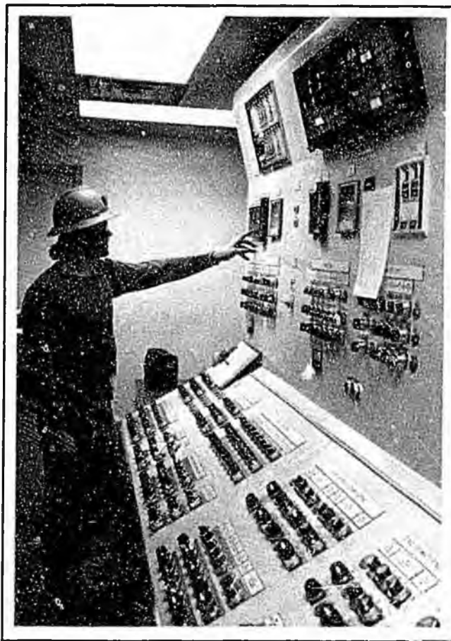
Mill Control Room at Greens Creek Mine
