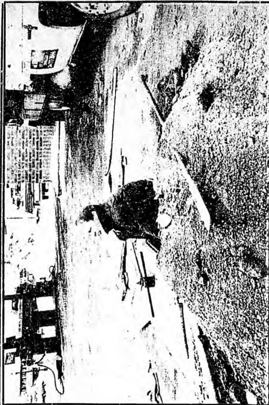
Kubalt Equipment and Service Company employee Terry Michels installs elbow joints in the submerged pump hole at Stremel's Quick Mart at the corner of Third and Lincoln Ave.
