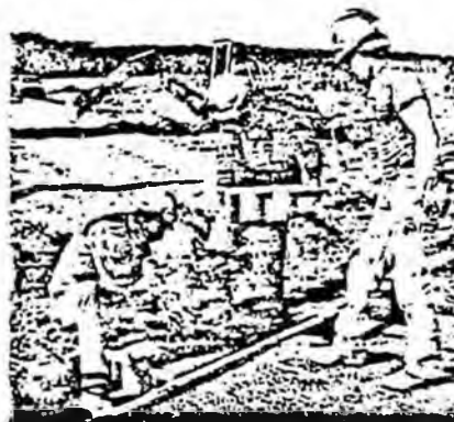
Maintenance workers installed a new, high technology material at railroad crossings that will provide a better crossing surface for the traveling public.
