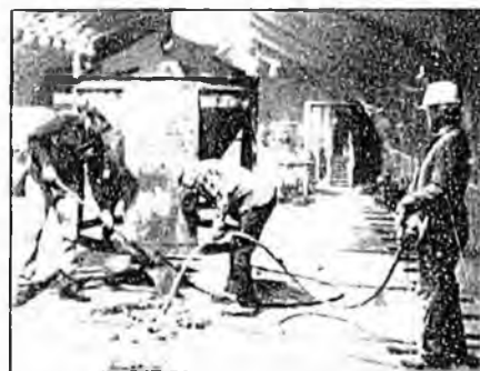
Crews quickly assembled 40-ft. by 30-ft. bridge sections in a large metal rib and fabric building at the project site. Eight prestressed concrete panels were grouted onto four I-beams for each 40-ft. section. Cutouts in the panels fit over Nelson studs welded to the girders. PN&D photo.
