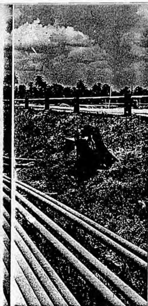
Pipelines bring oil to the outstation at Obagui in Nigeria—one of the world's leading oil producers.
