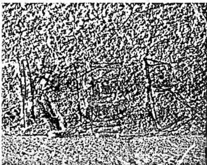
Friable Material That Has Been Scraped
