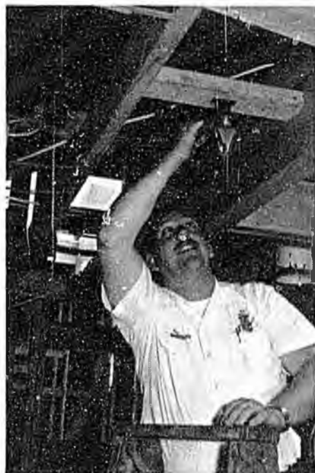
Inspector Ed Harrod of the San Clemente Fire Department checks a sprinkler system that uses polybutylene pipe.
