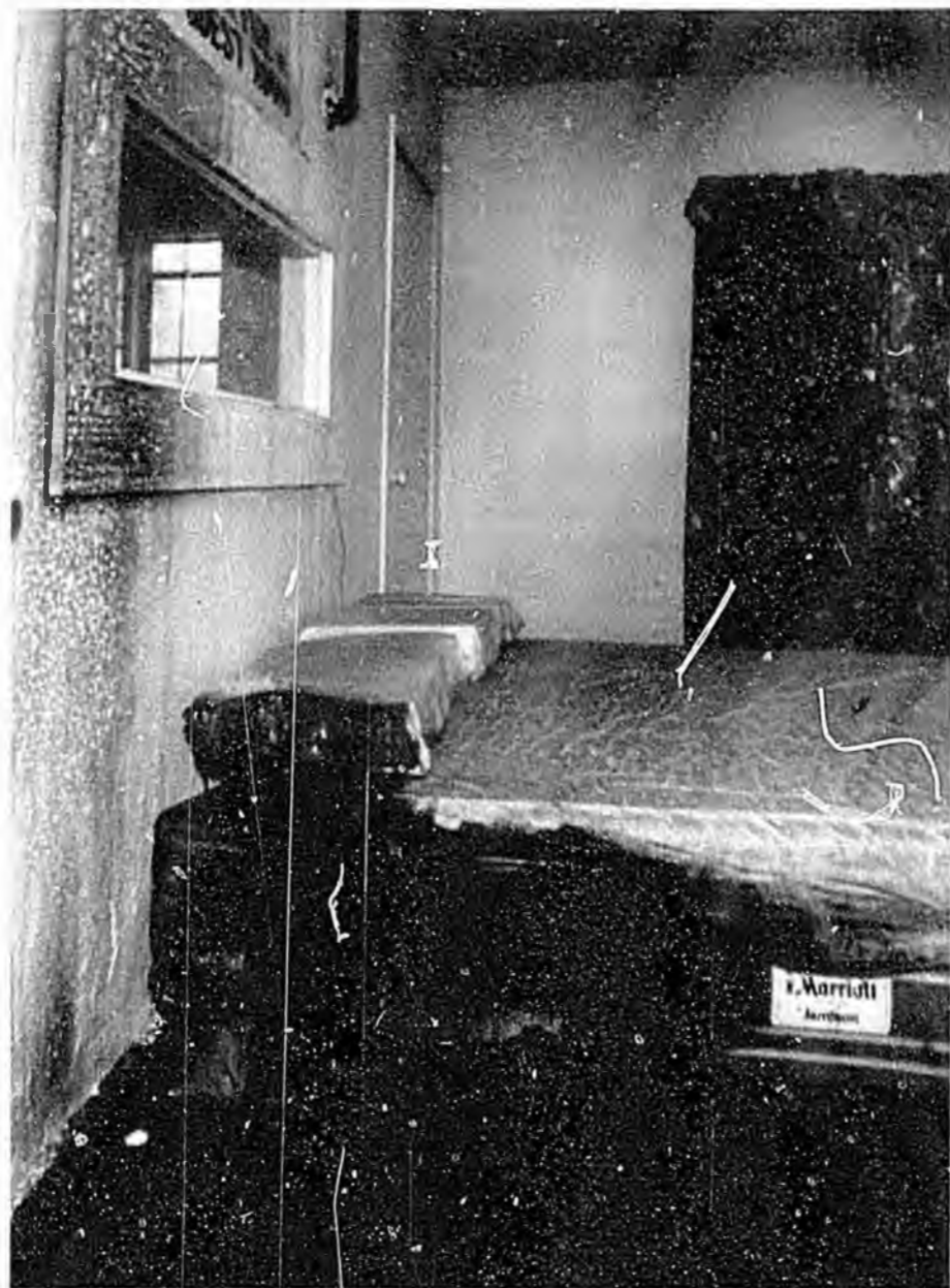
Detail of the damage to the bed and wall following activation of the sprinkler system.
