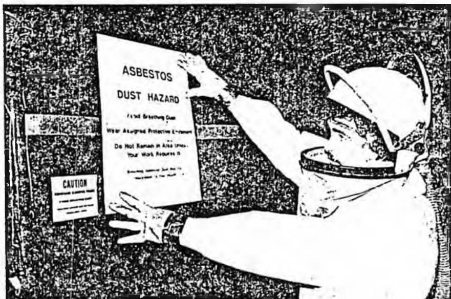
Schools are required to post warnings wherever friable asbestos exists. When asbestos is removed, areas are quarantined and workers wear protective suits.
