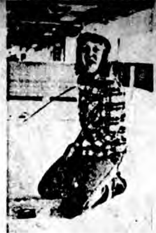
Cynthia Thomas, an 80 per cent apprentice of Local I.B.E.W. 1547 is caught in the act of stringing electrical wire.
