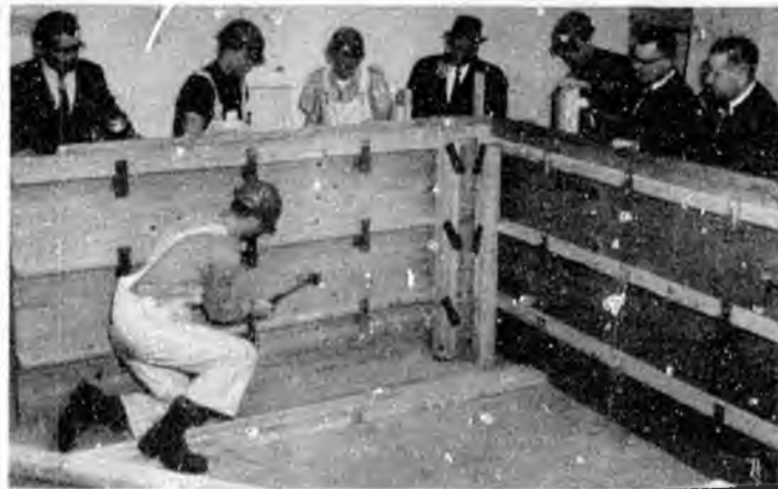
Concrete wall forms erected by apprentices as part of their related training.
