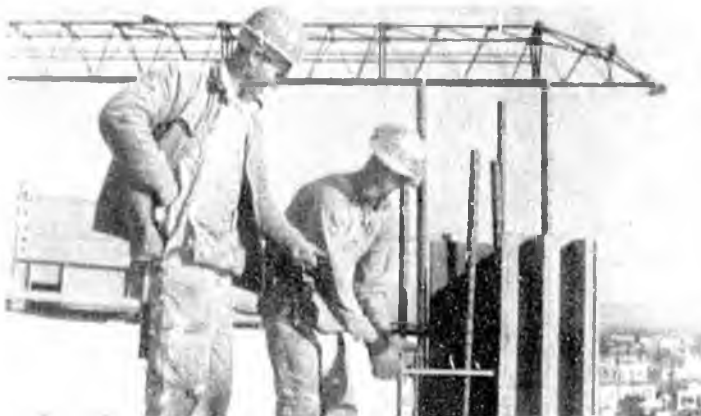
A carpenter apprentice, working with a journeyman carpenter on a reinforced concrete form job.
