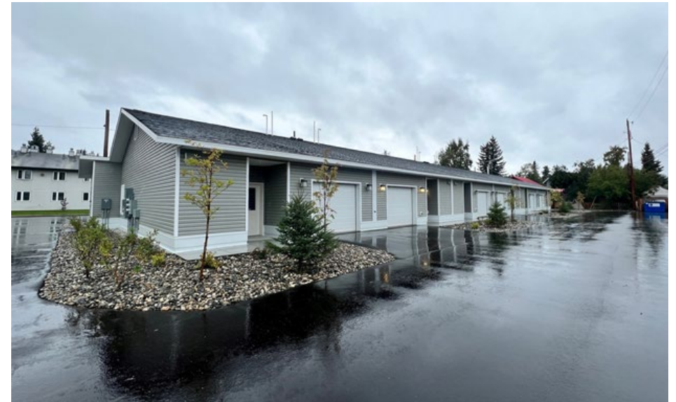
Alaska Corporation for Affordable Housing is constructing 58 new units in Fairbanks. Completion date: Sept. 2024.
