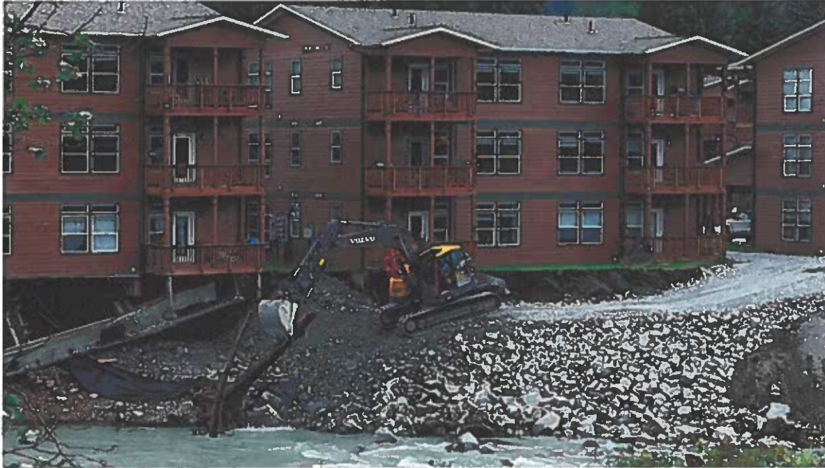
Workers removed debris and added rock fill along the bank at Riverside Condominiums on Aug. 8, 2023. (Andres Javier Camacho/KTOO)
