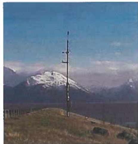
RWIS Installation at Bird Point, Jack Stickele, ADOT&PF
