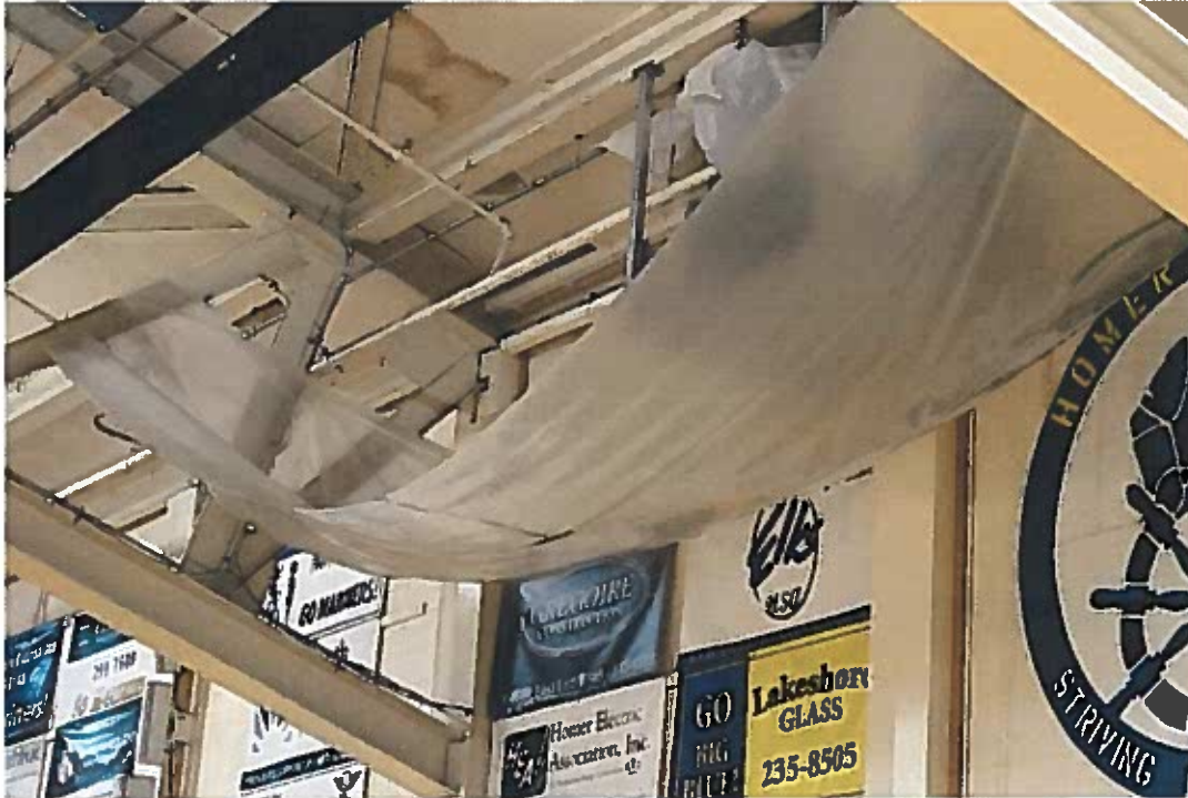
A large tarp hangs in the Homer High School gymnasium to catch water leaking through the roof at the school in Homer, Alaska. (Photo courtesy Doug Waclawski)
