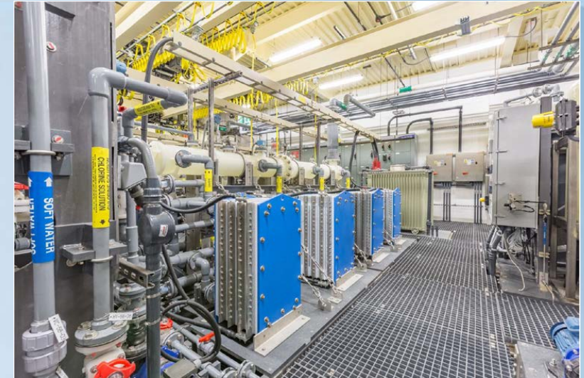
New Asplund Disinfection System
