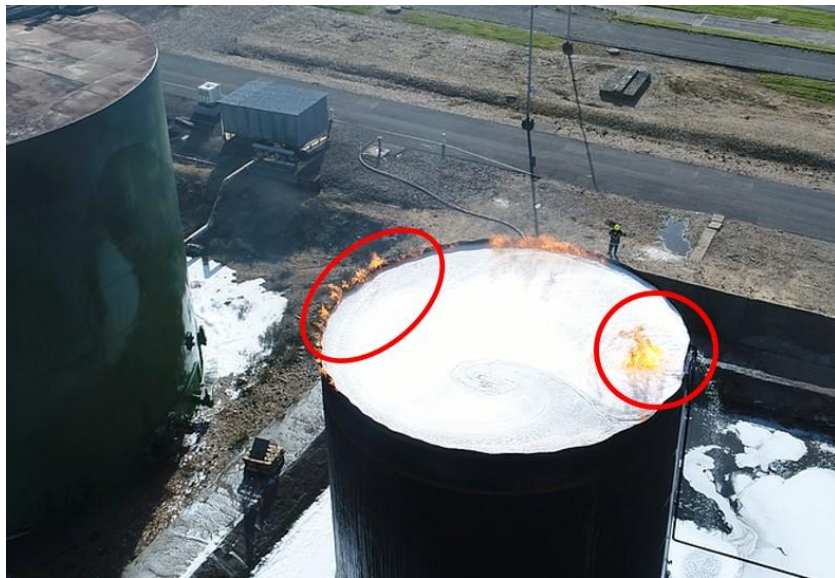
Poorer quality foam with system application. Note issues sealing at edges and control of impact point.
