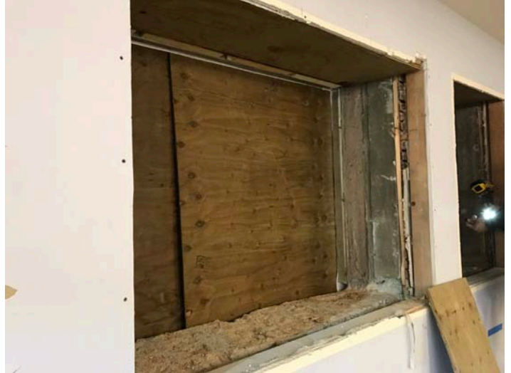
View of typical window sill in Library. Sills require grouting to fill voids for proper window receiver shimming and form smooth transition to support scheduled exterior and interior sill and flashing.
