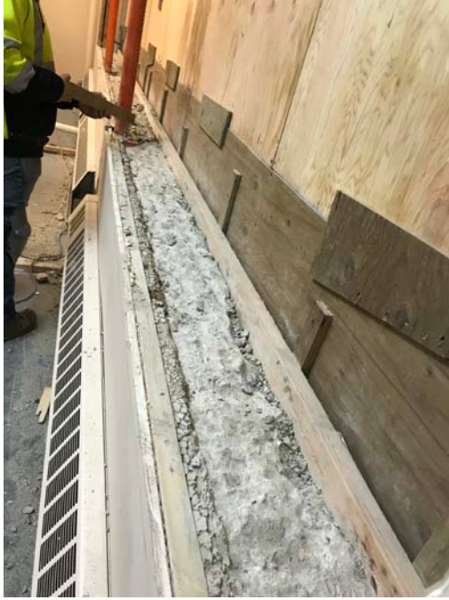
View of typical West addition sills along Main Street. Sills require grouting to fill voids for proper window receiver shimming and form smooth transition to support scheduled exterior sill flashing.
