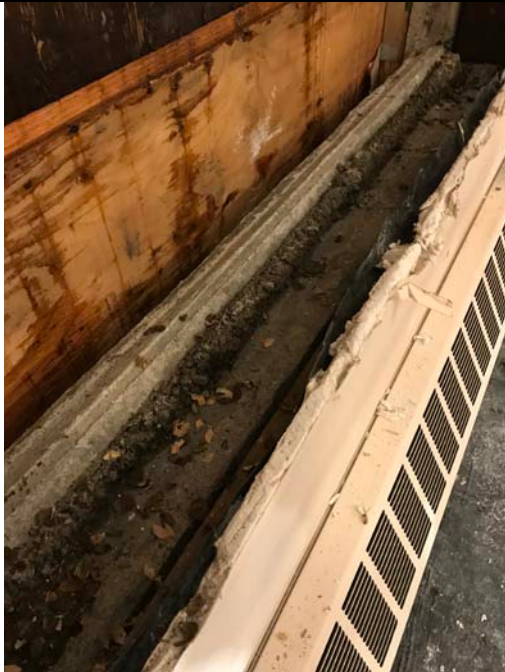
View of typical north and south window sills under abated wood window bucks that became the wood grounds for original wood window rough opening. Sills are heavily impacted by air pockets, unconsolidated concrete and concave voids. Sills throughout the 1927 and 1961 work require grouting to fill voids for proper window receiver shimming and form smooth transition to support scheduled exterior and interior sill and flashing.
