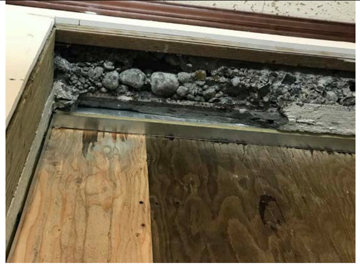
View of the typical window head encountered along the third floor of the 1927 structure. The concrete that was placed at the window bucks and appears to not have consolidated around the lower rebar. The condition of the heads varies due to the size of the aggregate used during this time.
