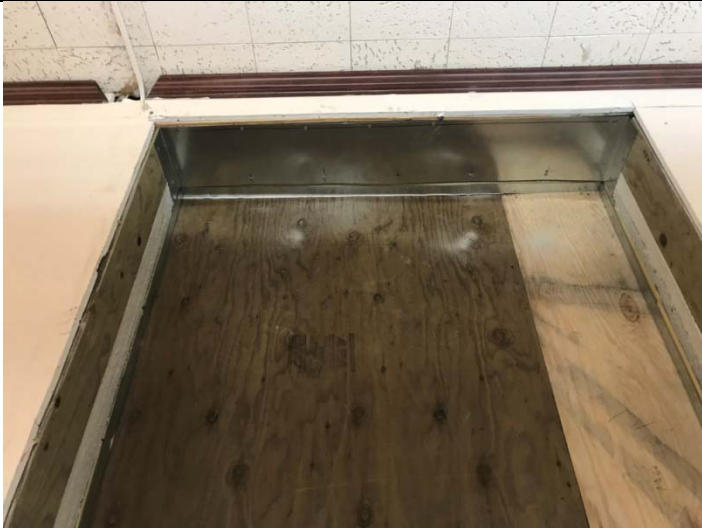
View of typical window head repair anchored into concrete at window heads and jambs.
