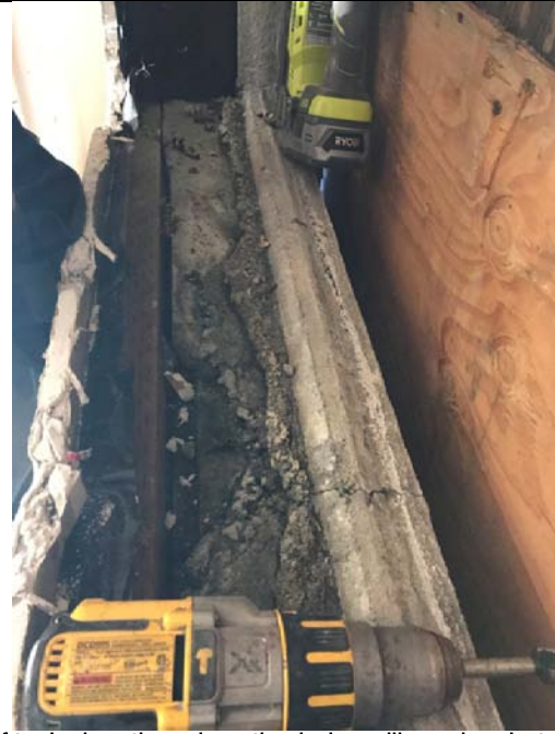
View of typical north and south window sills under abated wood window bucks. This condition of unconsolidated concrete under the window bucks (wood grounds) is present at all floors and window openings that have been demolished.
