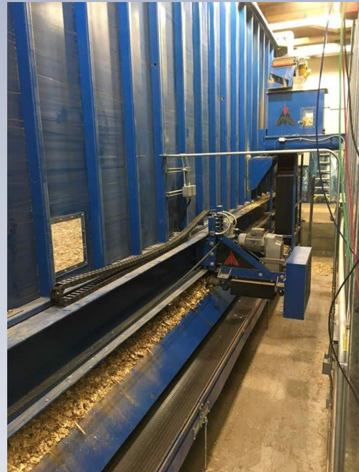
Chip Auger and Conveyer to Day Bin and Boiler
