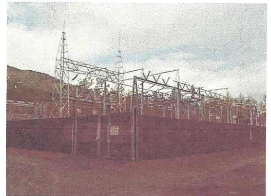
In 2013 thieves stole copper ground wires from the Daves Creek Substation near Cooper Landing.
