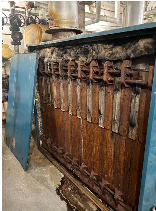
Kenny Lake Boilers - Copper River School District
