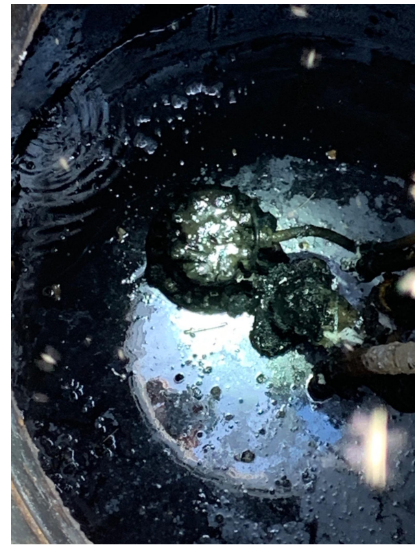
Flooded septic tank due to pump failure - Lake and Peninsula Borough School District
