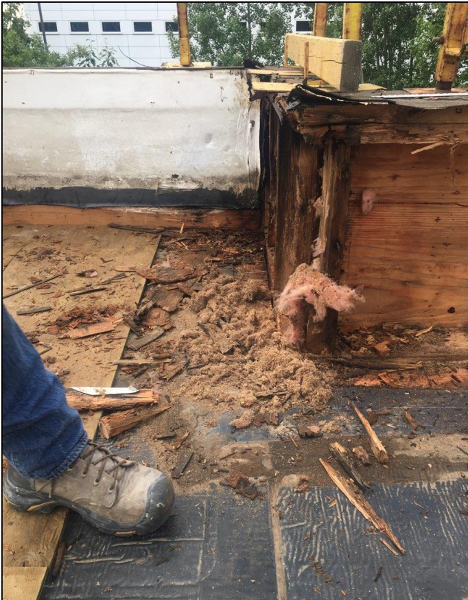
Rotted roofs cause continuous reactive maintenance and empty units at Cutler
