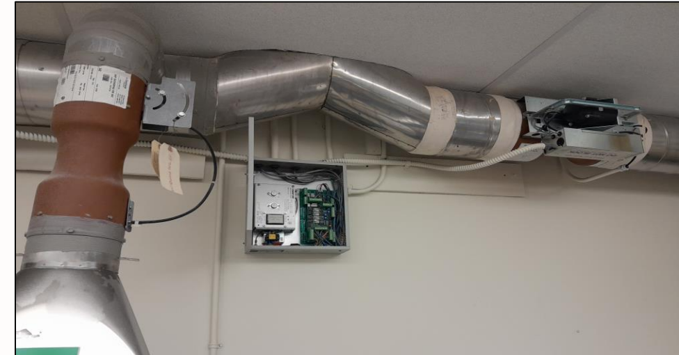
Unsafe lab conditions due to failed ventilation component
