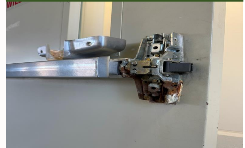
Parking Garage – Egress Door Hardware Corrosion
