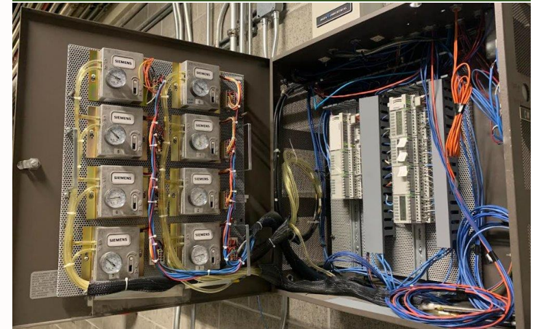
Outdated Pneumatic Controls
