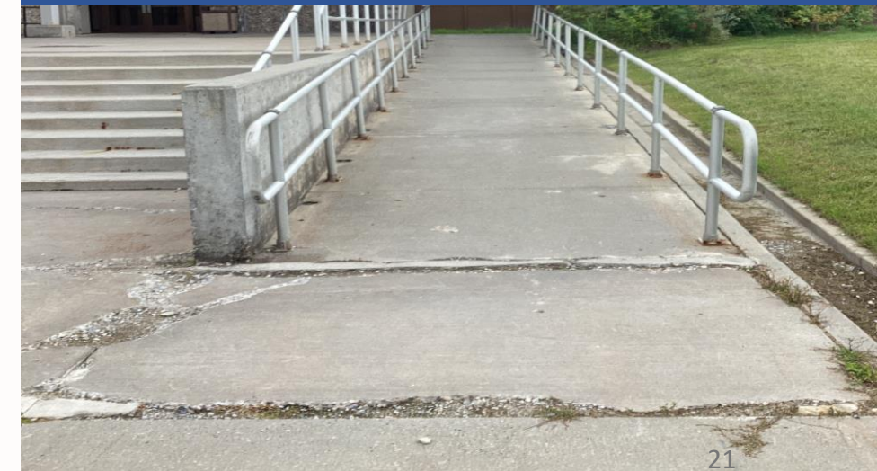
Broken/Uneven concrete preventing ADA Access up ramp
