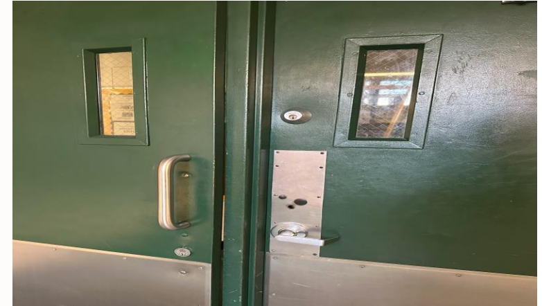
Avis Alaska Sports Complex – Door Hardware Failure
