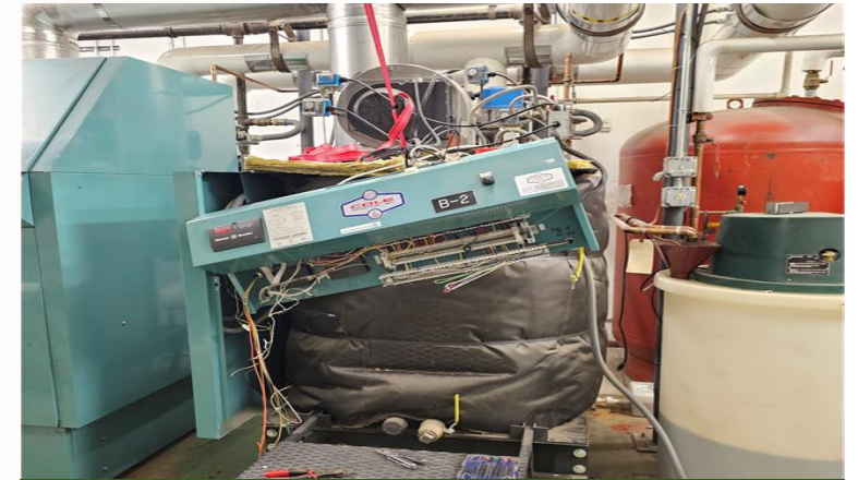
Boiler Failure and Repair
