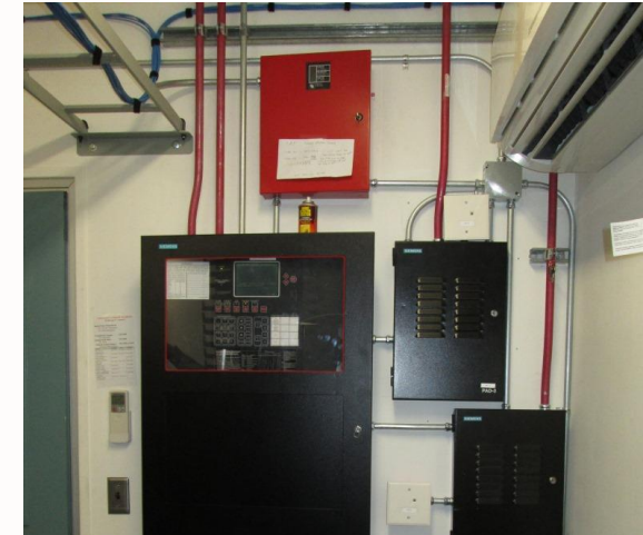
Fire panel malfunction requiring fire watch or building closure
