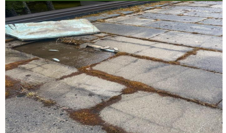
Campus Center Roof and Saturated Insulation
