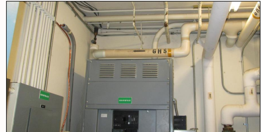
Electrical Panel exposed to aging pipe systems leads to failure and disruption to operations
