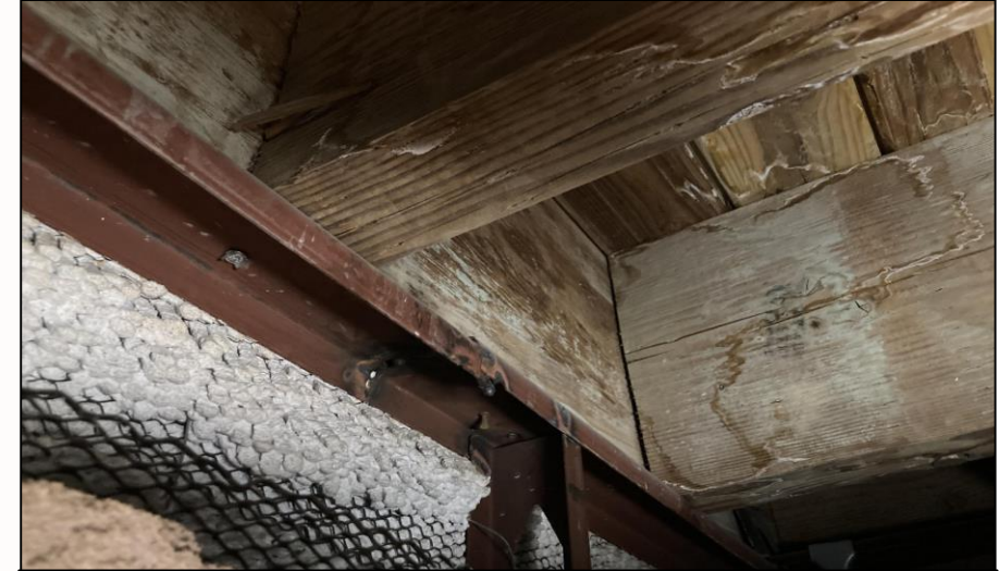
Salisbury: Wood structural framing creates a fire hazard
