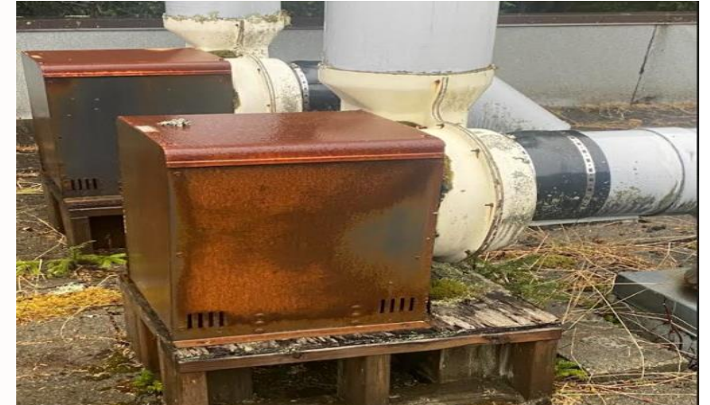
Vo-Tech Lab Circulation Pumps
