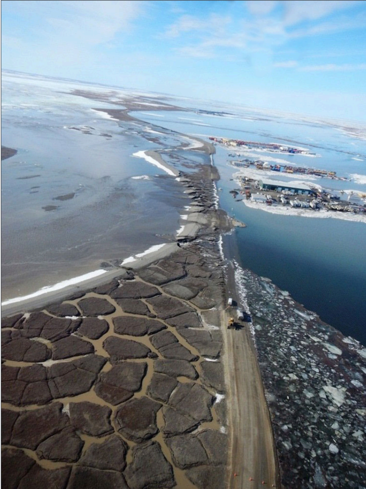
Catastrophic flooding in 2015 shut down the Dalton Highway for 28 days, prompting two state disaster declarations to be issued. Photo taken in May 2015 by Alaska DOT&PF staff
