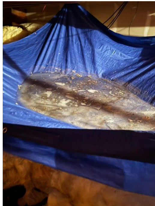
Ice in tarps - McGrath School attic
