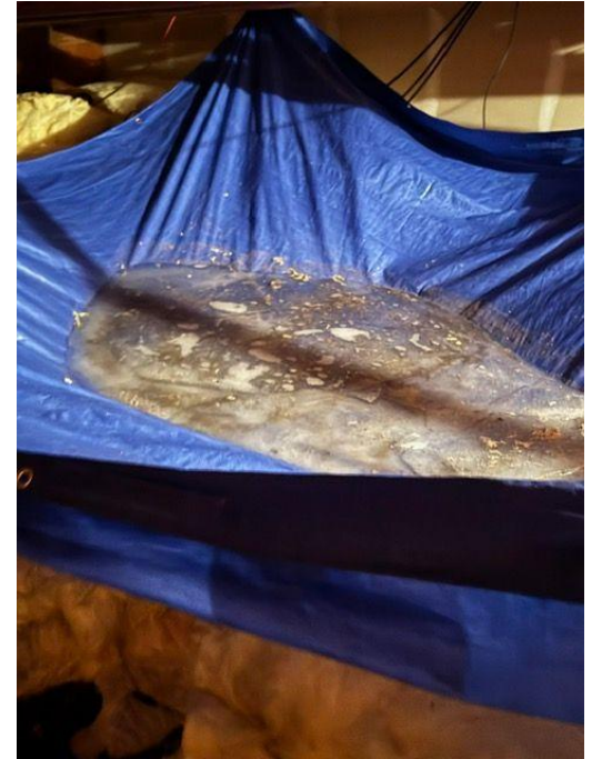
Ice in tarps - McGrath School attic
