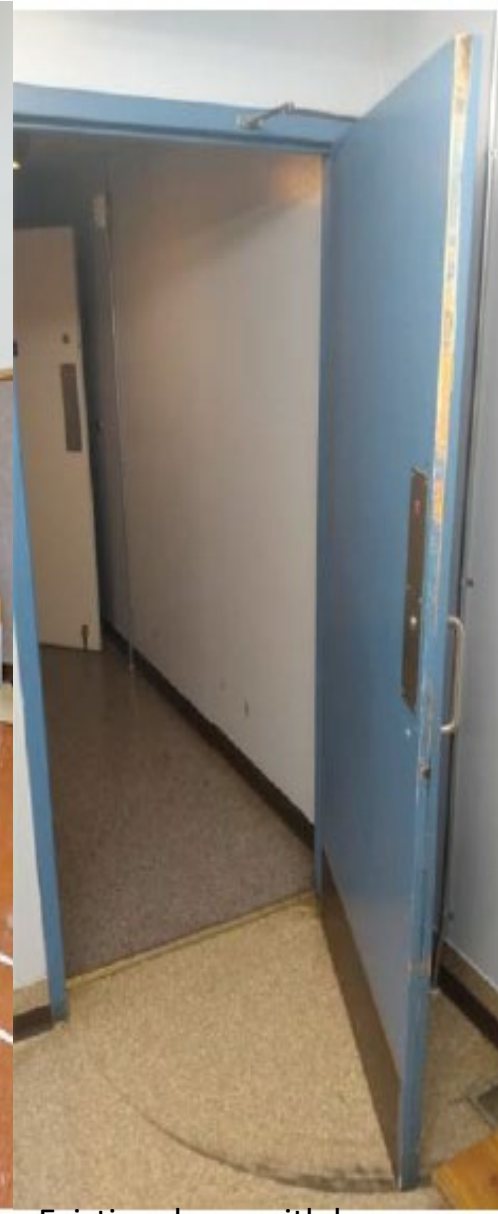
Existing doors with loose hinges – A Project currently on Major Maintenance List
