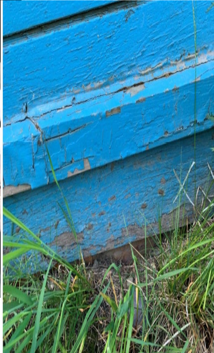
Siding Condition at Foundation – A Project currently on School Construction List
