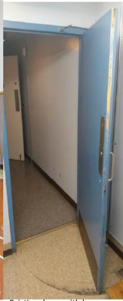
Existing doors with loose hinges – A Project currently on Major Maintenance List
