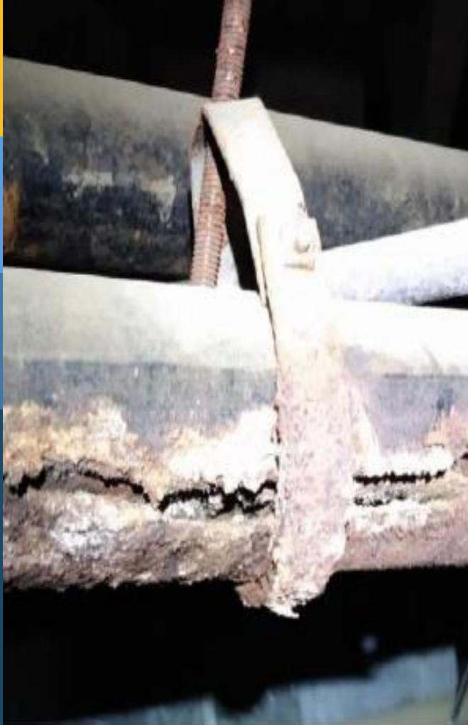
Broken Waste Pipe – A Project currently on Major Maintenance List
