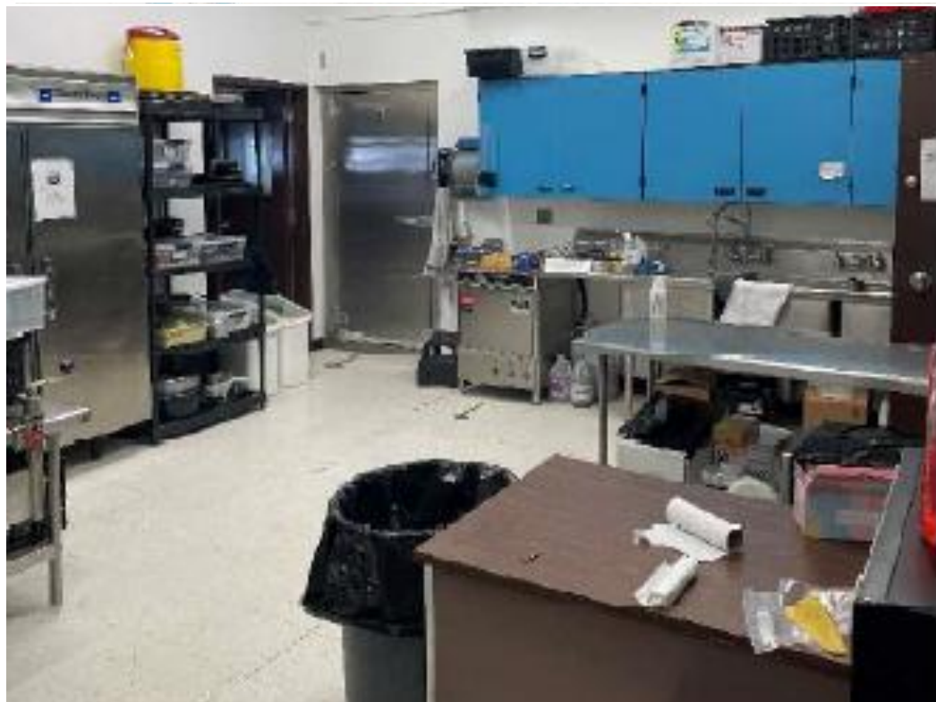
Compartment sink, walk-in freezer, upright refrigerator, desk, and entrance into dry storage – A Project currently on the Major Maintenance List
