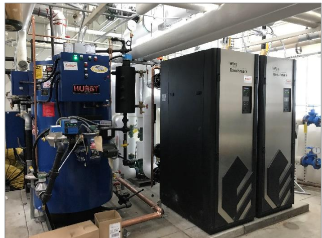
EHL New Main Heating & Steam Systems
