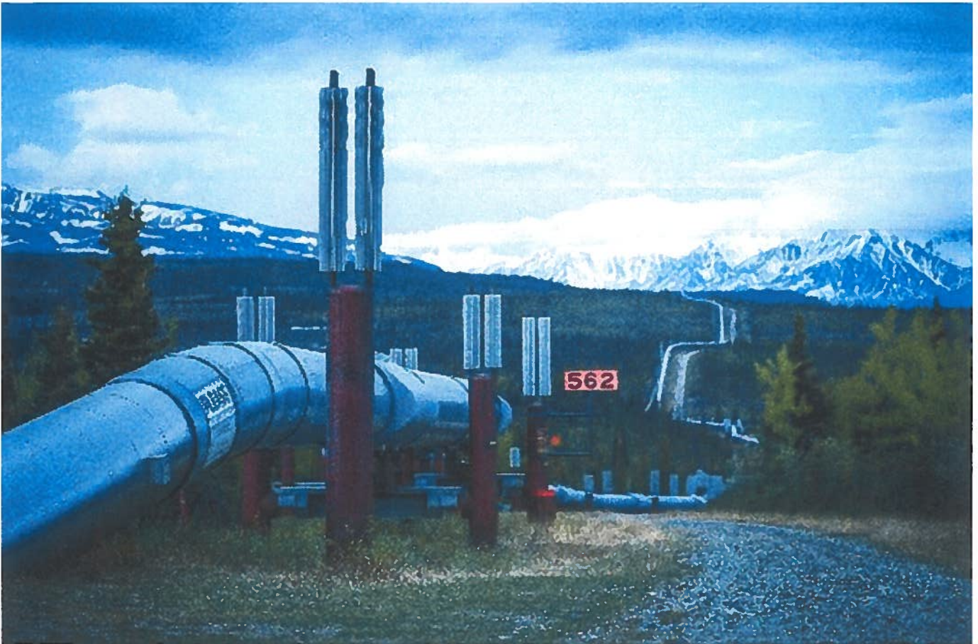
The trans-Alaska oil pipeline as seen near Delta Junction in June 2013. (Loren Holmes / ADN archive 2013)
