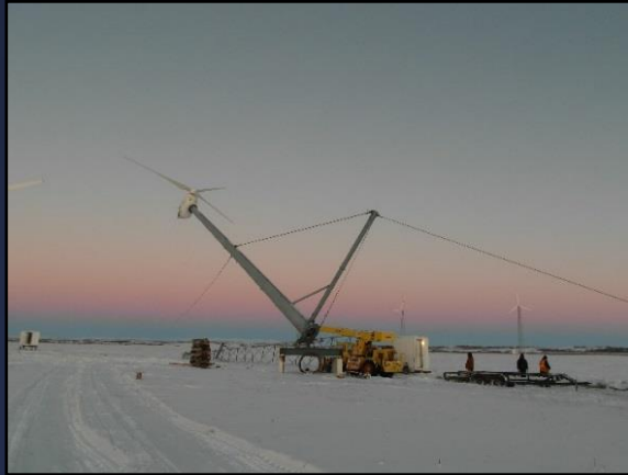
Arctic Field Testing of Eocycle Wind Turbine
