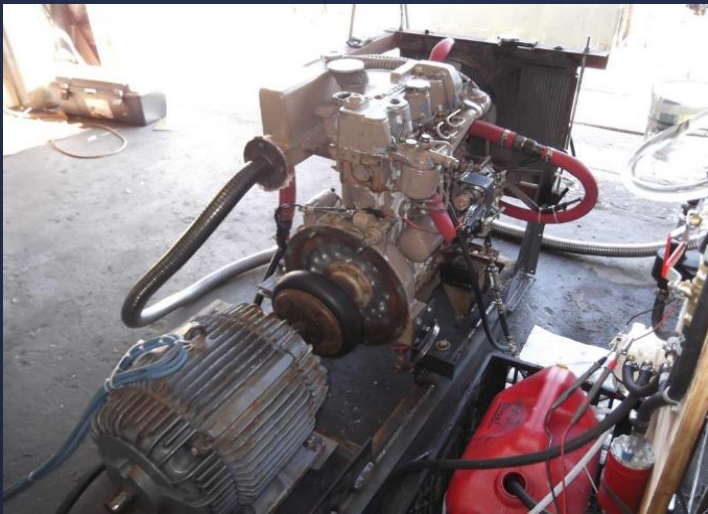
Modified 15 kW Genset
