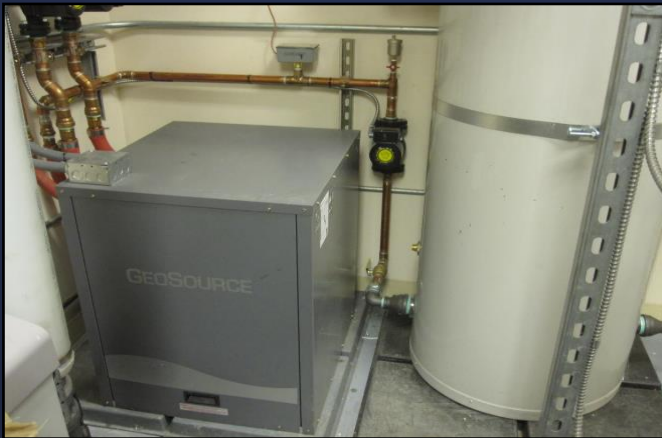
Installed 6-ton Heat Pump
