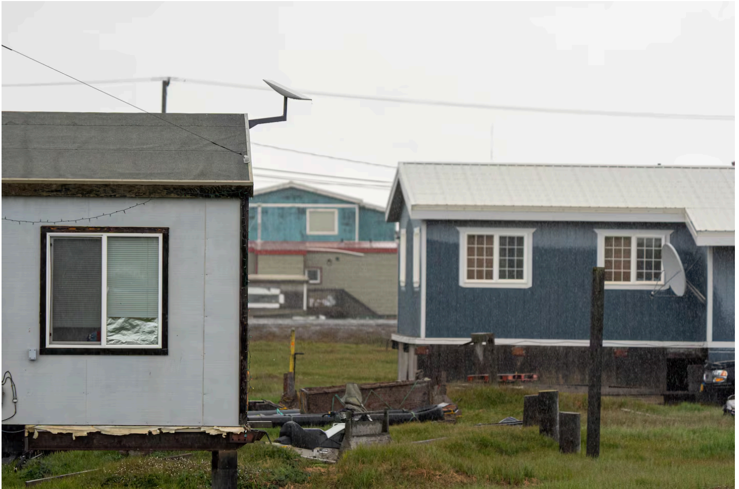
A Starlink dish is installed on a house on Saturday, Aug. 10, 2024 in Utqiagvik. (Loren Holmes / ADN)
